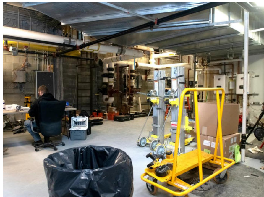
The heating, ventilation and air conditioning room of The Palace Theatre.
